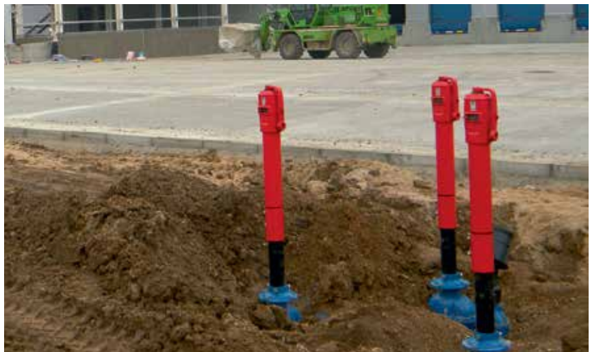
AVK series 34/00 post indicators for fire protection at FM Logistics - Petresti, Romania.
